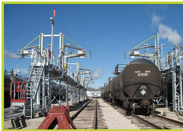
Wagon Gantry Loading/Unloading
